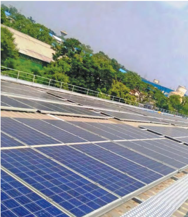
2 MW Industrial Roof Top in Chennai, Tamil Nadu
