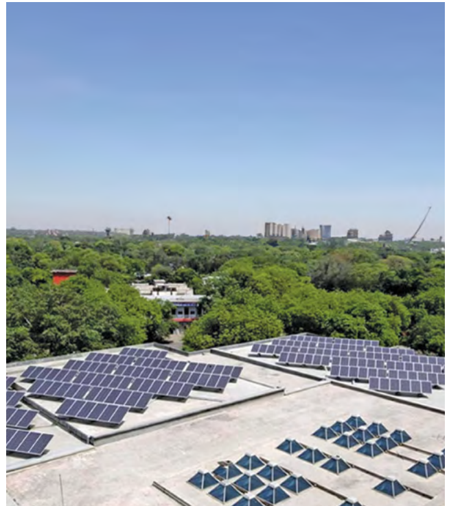
80 kWp Grid Tie SPV Plant, Indian Parliament House, New Delhi
